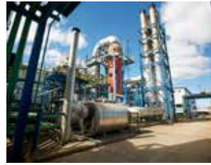
Mali Heavy Fuel Oil Power Plant
